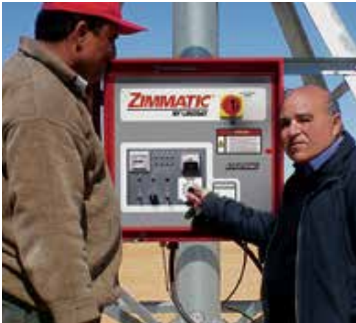
BASIC Control Panel
